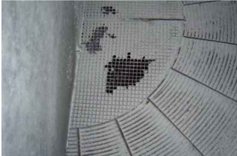
FIGURE 1. COMPLETE BLOCKAGE OF A FAN WITH CIPC AFTER RECIRCULATION OF FOG AT FULL SPEED
