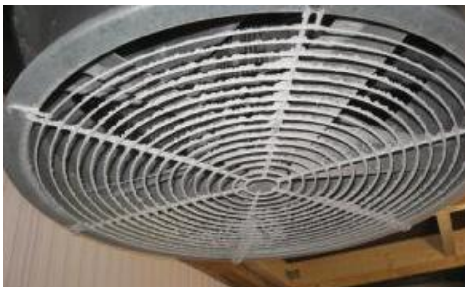
Figure 7. Deposition of a white powder on fan guard following CIPC application.
