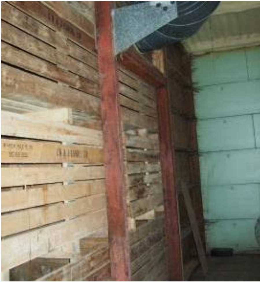
Figure 3. Fixed, open-fronted ‘Strawson wall’ against which boxes were stacked to create an ‘open suction’ circulation system in Store C6.
